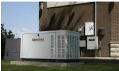
Generator For Common Area
